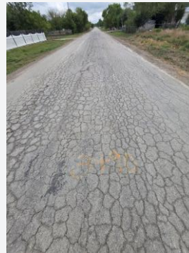
Figure 9 Spruce Street Existing Road Conditions Cracked Marked 3+90
