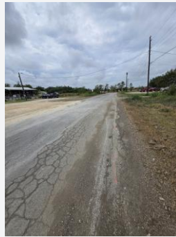
Figure 7 Spruce Street Existing Road Condtiion
