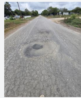
Figure 8 Spruce Street Surfacing Pothole
